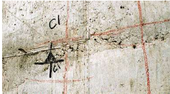
Figure 1: Cold joint formation (Volz, 2007).
